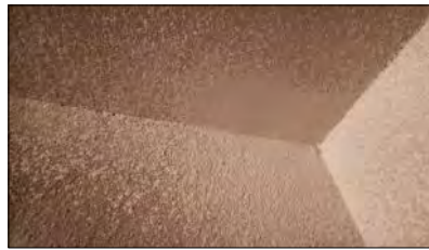
Montrose mom Dustie Johnson took this photo of a corner with mold problems in an American Village rental. Courtesy photo.
