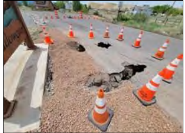
An emergency culvert repair has become necessary at the Meadowgate Subdivision in Montrose, where sink-holes have developed in the roadways. City of Montrose courtesy photo.
